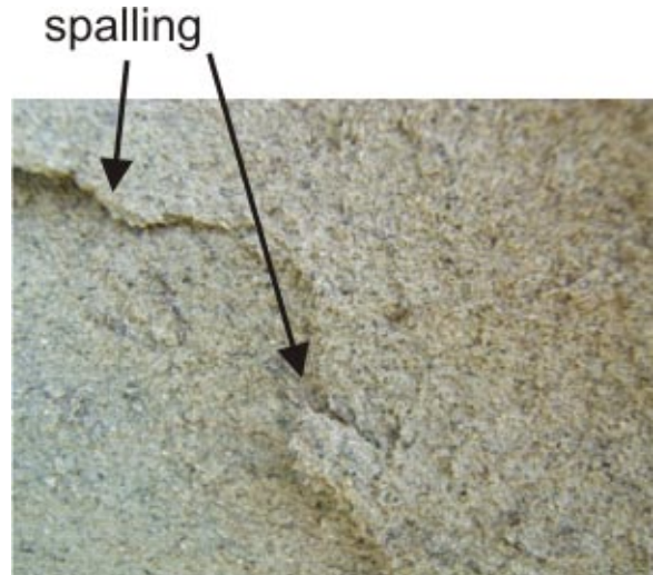
Below: Sandstone on the back walls of galleries on Gabriola also spalls. Although not visible in this photograph, salt is often found on the undersides of the flakes.
