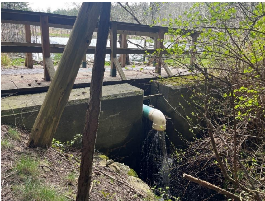
Photo 3-7 View of the syphon at the downstream side of the concrete weir on April 4, 2024.
