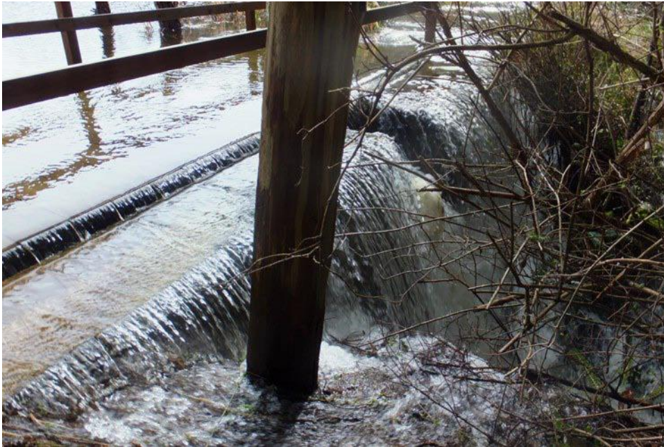
Photo 3-8 View of the syphon at the downstream side of the concrete weir on March 10, 2016 (photo by Gabriola Streamkeepers 2017).
